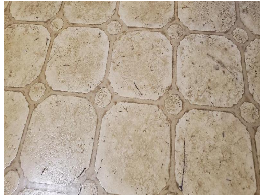
923-3 Rolled Flooring (20% Chrysotile) Mastic Interior Kitchen (approx. 150 sq. ft.)
